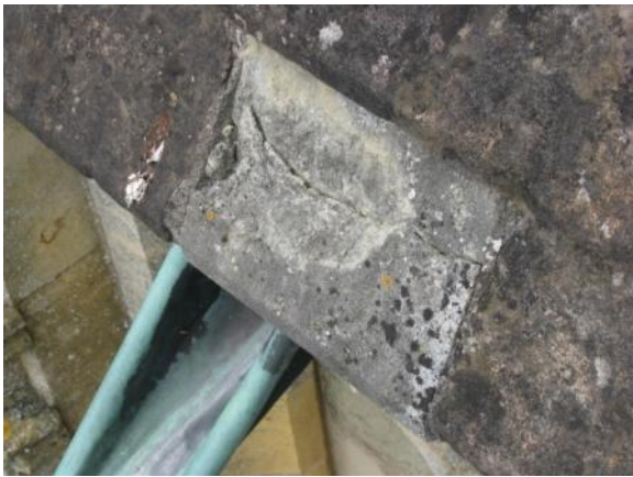
Cracked and decayed section of tower string course
