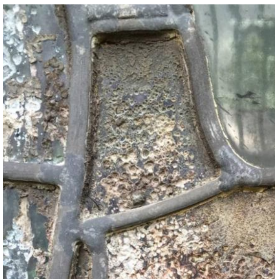
Example of corrosion from the exterior side of a window in St Anne's Chapel. Different levels of corrosion are visible, as well as extensive pitting with a mixture of dirt and corrosion products
