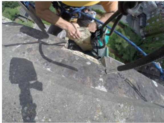
Cracked section being removed for safety
