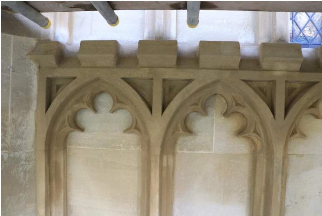
Figure 22: Sheltercoat (still wet) applied to a section of the parapet after cleaning and repair
