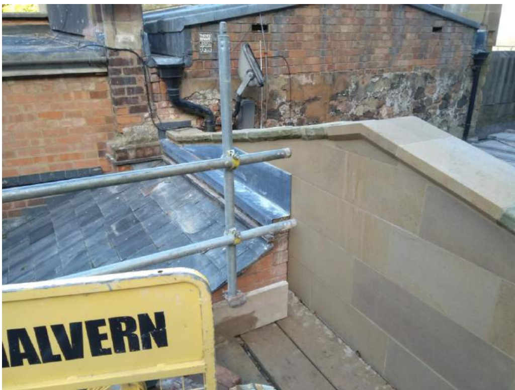
Figure 8: The completed gable of the wall viewed from the hotel side. Note the new flashing above the 'lean-to' shown in figure 2
