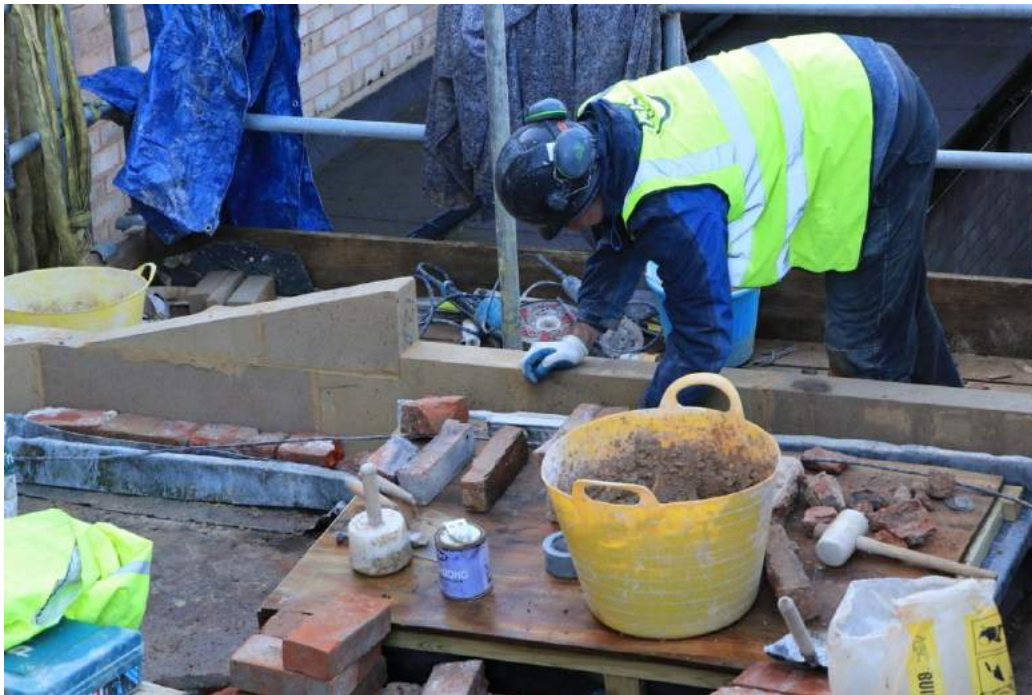
Figure 7: Rebuilding the gable of the West Wall and its brick face (viewed from the aisle roof)
