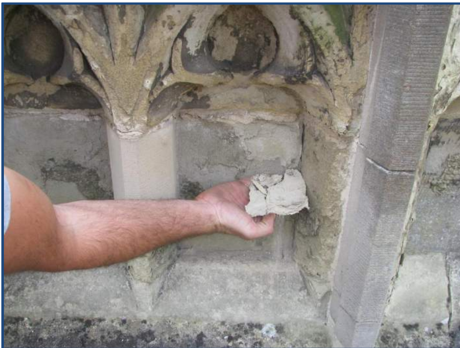
Figure 12: Dirty and decaying stone in the parapet.
